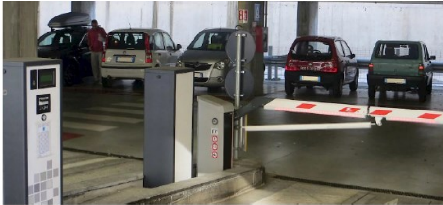
Figure 4. Entrance and exit parking barriers
