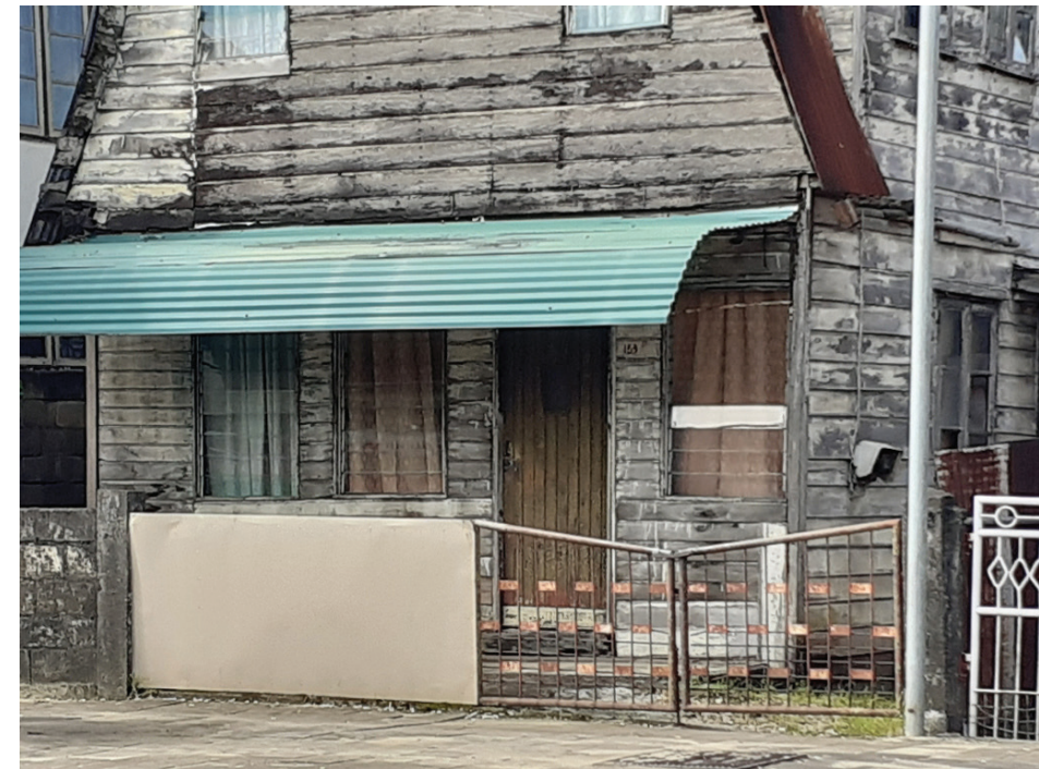
Figure 29. Non Contributing Alteration
