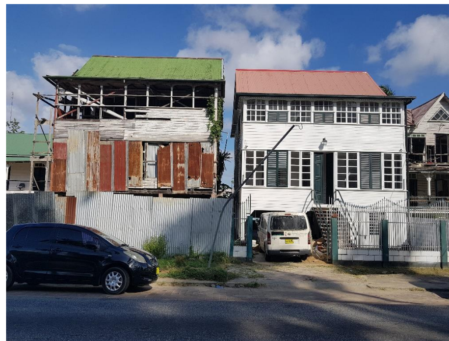
Figure 48 – Fire is the most serious risk in the historic inner city. Recently restored homes adjacent to high-risk abandoned structures makes insurance impossible (Eppich, 2019)
